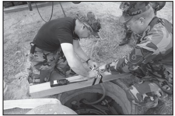
Top: SSgt. Marinko Lemut, 270EIS (left) and MSgt John Cass, 111CF (right) work on cable pulled across the flightline.
